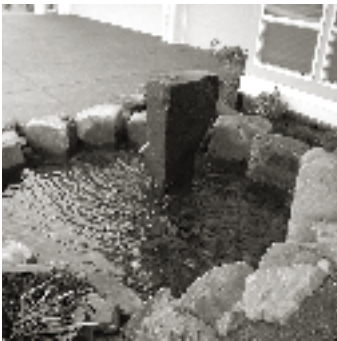
Above top to bottom: One of the team drilling a bronze basalt column using a 30 lb. pneumatic drill. Completed center stone feature with top of stone honed to disburse water evenly to all sides.
